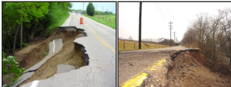
Canal Road wash out from flash flooding, July 2001.
