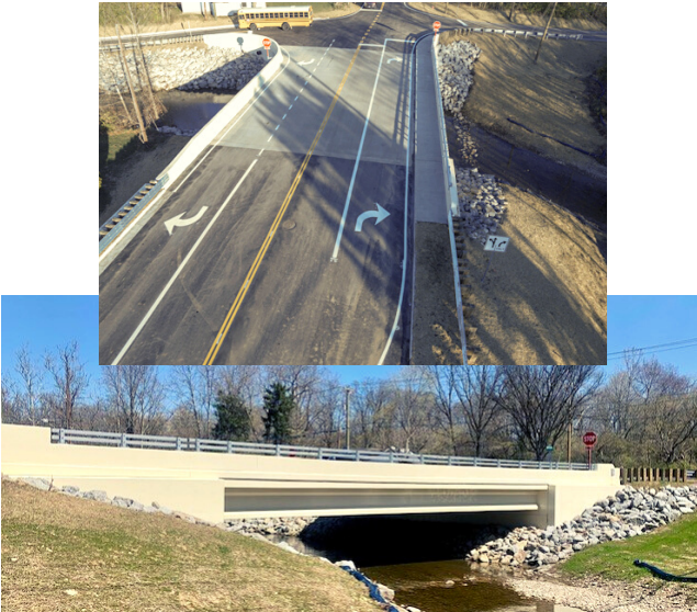
HAMILTON MASON ROAD BRIDGE #7.49 Bridge Replacement Total Construction Cost: $1,687,887.00 Funding: State, BCEO
