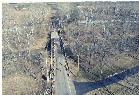
ELK CREEK ROAD BRIDGE #5.004 Bridge Rehab for a one-lane bridge Total Construction Cost: $183,289.00 Funding: BCEO
