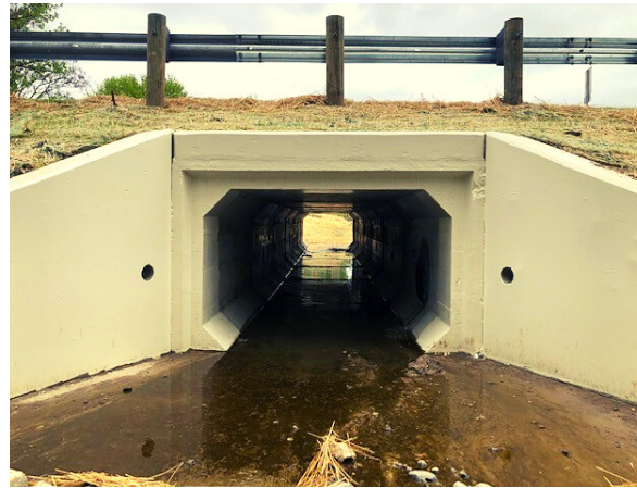
MIDDLETOWN GERMANTOWN ROAD BRIDGE #0.393 Bridge Replacement Total Construction Cost: Included in the multi-culvert contract cost (next page) Funding: BCEO
